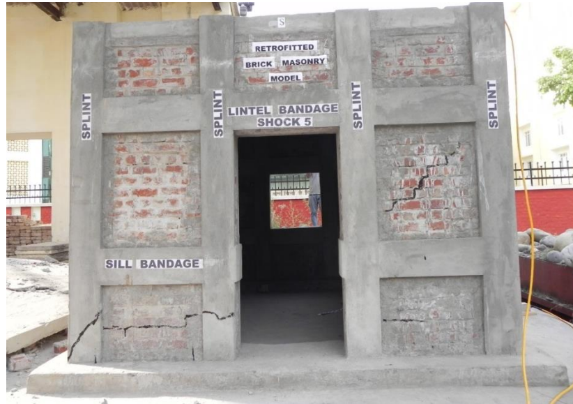
Fig. 5 Front view of shock-table platform showing view of minor cracks developed in retrofitted models after shock 5 on southern side
