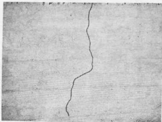
Fig. 10. Crack in the abutment of a road bridge.
