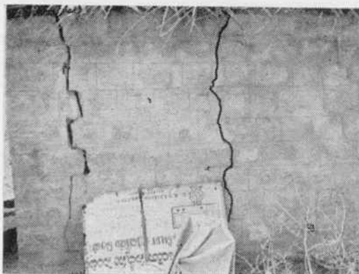
Fig. 9. Widening of cracks in a stone masonry wall.
