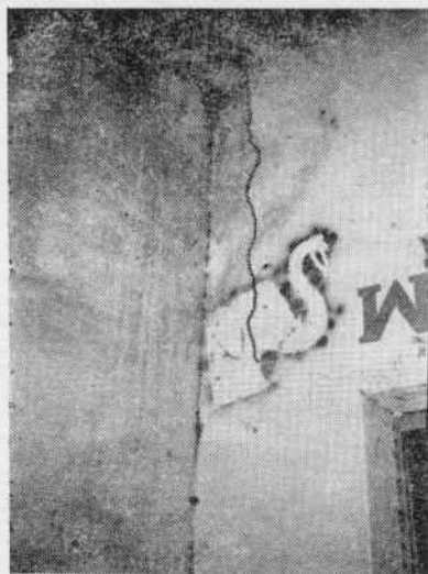
Fig. 14. Cracks in the wall of a flour mill in Kowthalam.
