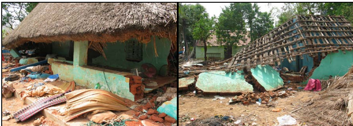
Fig. 7 Collapse of brick masonry houses in Kudukuppam (Villupuram)
