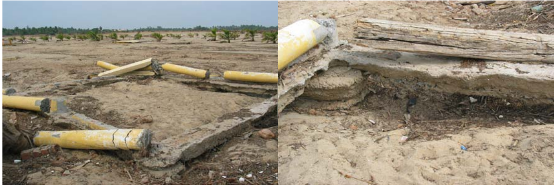
Fig. 16 Foundation of collapsed Sri Karneshwara Natraj Temple (Kudukuppam) (only isolated footings under the columns were used)
