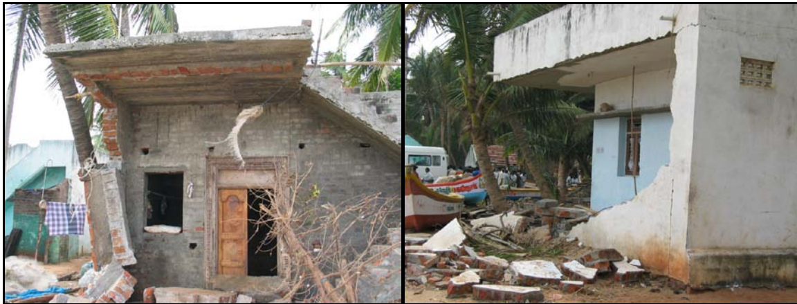
Fig. 6 Collapse of compound walls of residential houses in Chinapattam (these walls protected the houses from damage)
