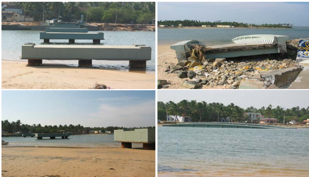
Fig. 21 Damaged bridge on the river Palyar in Keelamanakudy: (clockwise from top left) (a) the substructure left after 4 spans of the deck got washed away; (b) a span washed away by about 20 m; (c) another span moved by about 50 m; (d) bare substructure (with 2 spans still missing)
