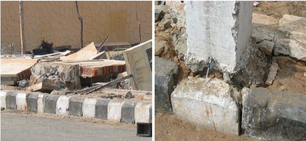
Fig. 4 Collapse of the compound wall of Madras Lighthouse (Chennai) (concrete posts of the wall separated; second figure shows that another post is displaced laterally by about 10 cm)
