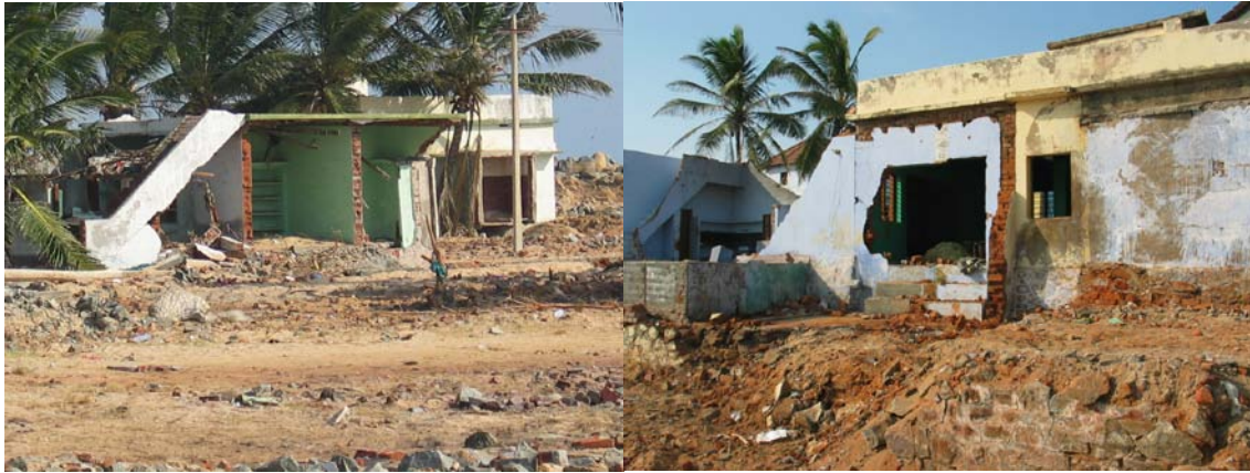
Fig. 11 Widespread damages to buildings in Meelamanakudy (Kanyakumari) (most of the houses were of brick masonry which performed poorly during the tsunami attack)
