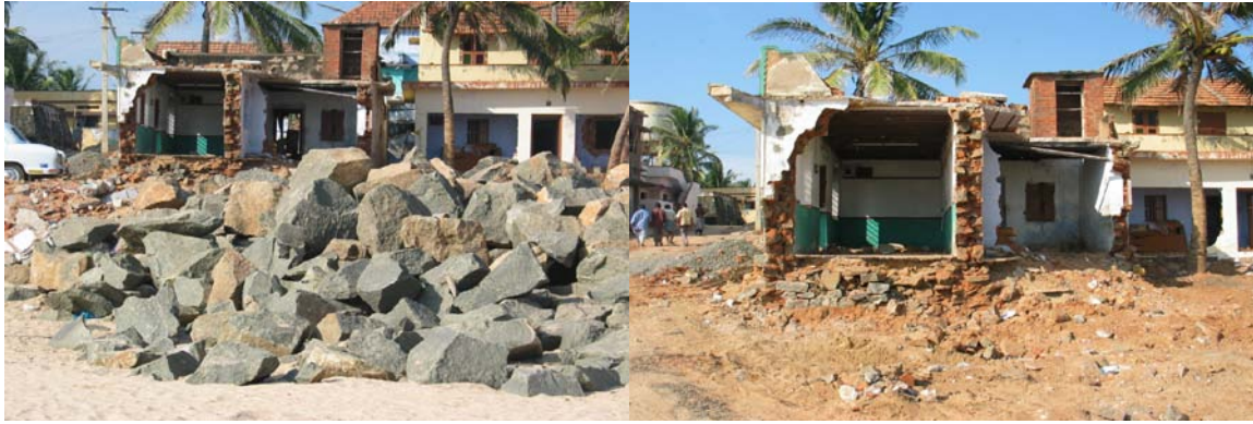
Fig. 20 Collapse of another building in Meelamanakudy (Kanyakumari) (close-up view of the collapsed front wall shows how vulnerable the brick masonry was to tsunami)
