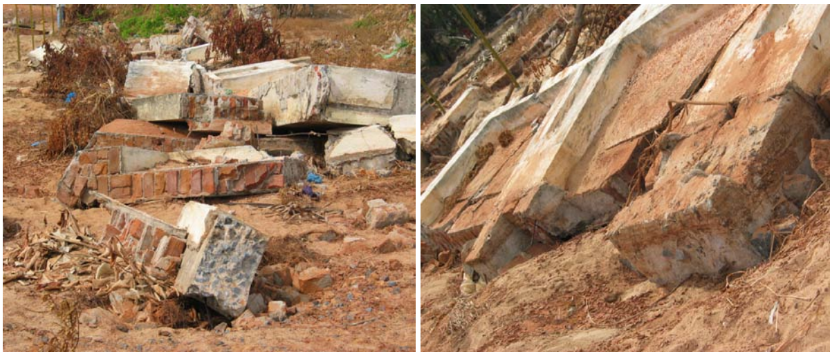
Fig. 5 Collapse of brick masonry compound wall of a school in Chinapattam (Pondicherry)
