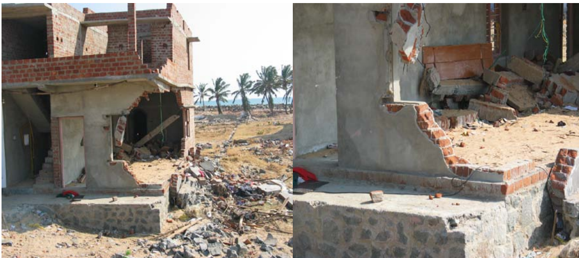
Fig. 10 Collapse of a brick masonry building under construction at Keelamanakudy (Kanyakumari)
