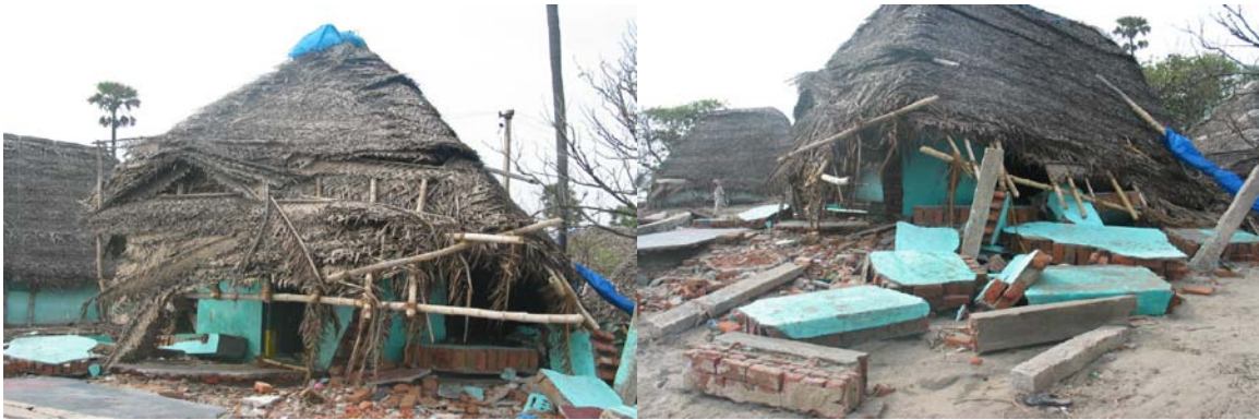
Fig. 14 Collapse of adobe houses in Nabiyar Nagar (Nagappattinam) due to tsunami
