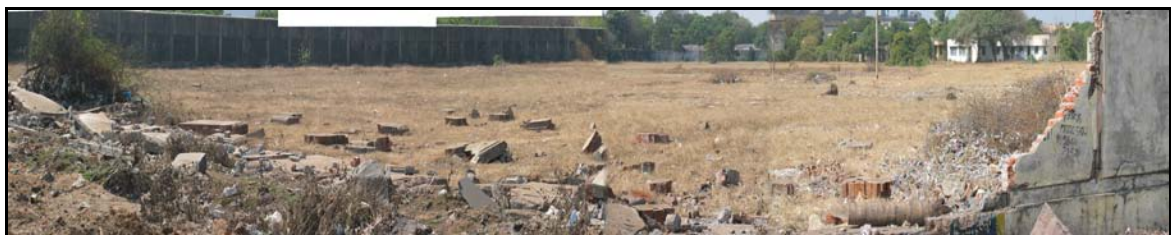
Fig. 3 The boundary wall of about 50 m length damaged in Cherain Nagar (Chennai)
