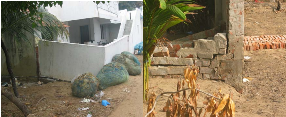
Fig. 8 Damage to boundary walls in Talenguda (Cuddalore) due to damage to brick masonry
