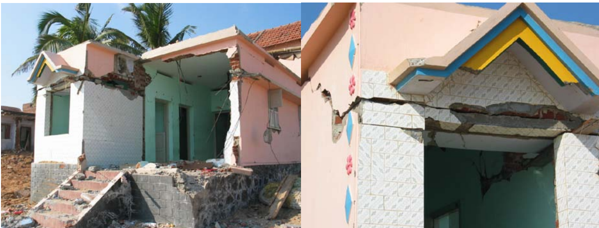
Fig. 19 Heavy damage to a building in Meelamankudy: (a) complete failure of joints at lintel band, (b) a close up view showing that there was lateral displacement of top part towards the right side
