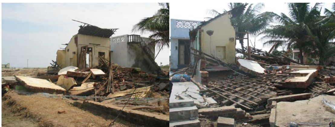
Fig. 12 Collapse of adobe houses in Kuddukullam village (near Cuddalore)
