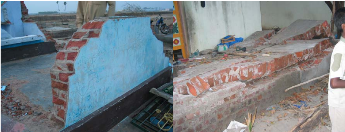
Fig. 9 Damage to brick masonry in Amman Kerapattu village (Nagappattinam) near Karaikal (even bricks used with lime mortar got broken here and wall collapsed)
