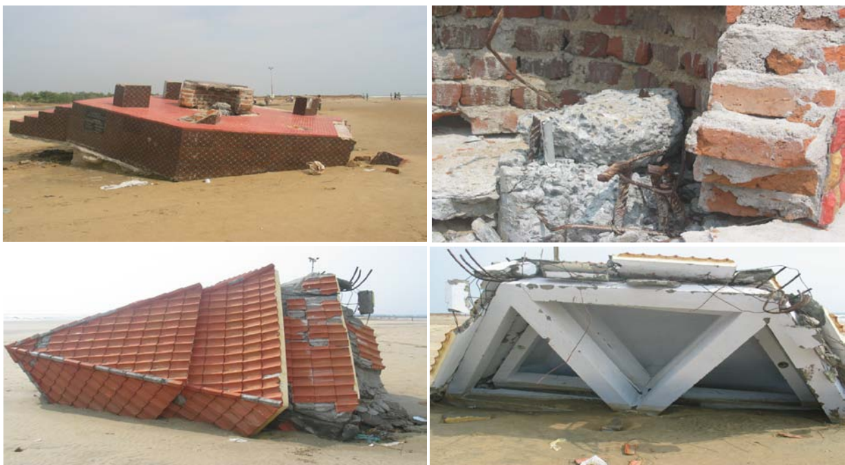
Fig. 17 Damage and collapse of a small monument in Devanam Kuppam (Cuddalore) (top left: tilted base due to settlement and erosion of soil; top right: heavy roof supported by a single column only; a collapsed RCC column without adequate reinforcement; bottom: displaced roof that toppled and moved away but remained relatively intact due to adequate reinforcement)
