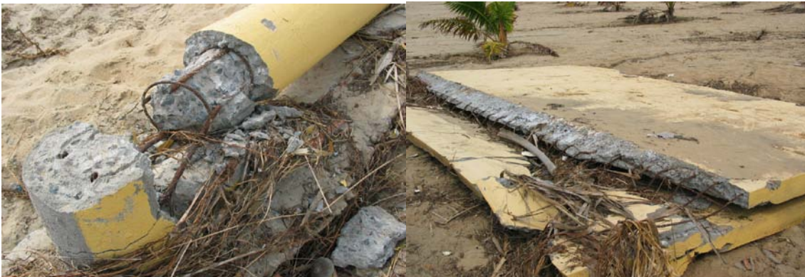
Fig. 15 Left: One of the failed reinforced concrete columns of Sri Karneshwara Natraj Temple, Kudukuppam (Villupuram); Right: Toppled roof, which moved few meters away
