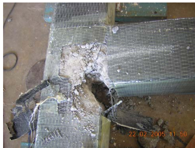
Fig. 13 Typical failure of beam-column joint with CFRP
