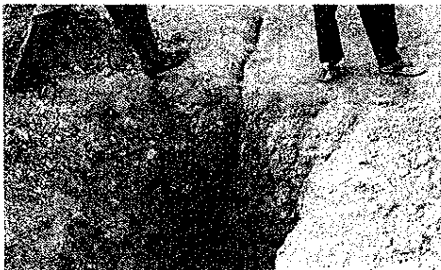
Fig 23 One meter deep fissure in left embankment of lower Terna dam, as confirmed by pit opening.
