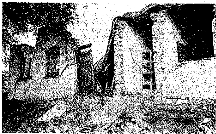
Fig 37 Collapsed school at Sastur.
