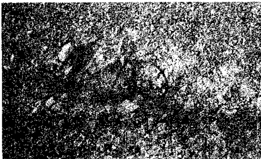
Fig 22 Slope failure of canal embankment at Ganjankheda.
