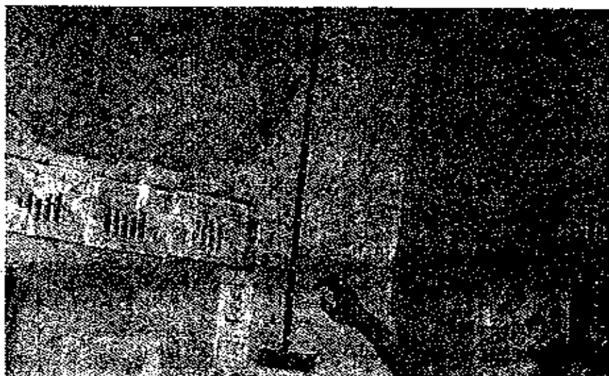
Fig 34 Doctors showing portion of a wall which developed cracks one year earlier, in the tremor of October 18, 1992. These were plastered subsequently, Rural Hospital at Killari.
