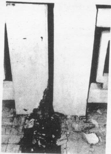
Fig. 7: Damage to Rail Post at Fixed End of Suspended Span
