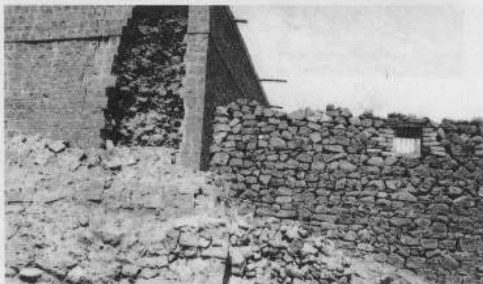
Fig.3 COLLAPSE OF OUTER WYTHE OF WALL TO FULL HEIGHT
