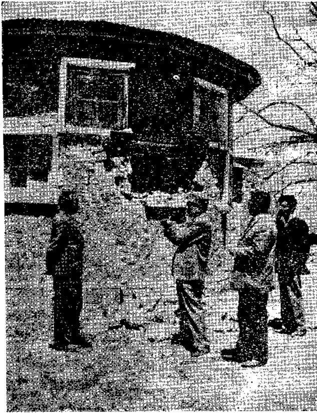
Fig. 31. Damage of Random Rubble Masonry Walls around Windows in B. D. O., Shangus.
