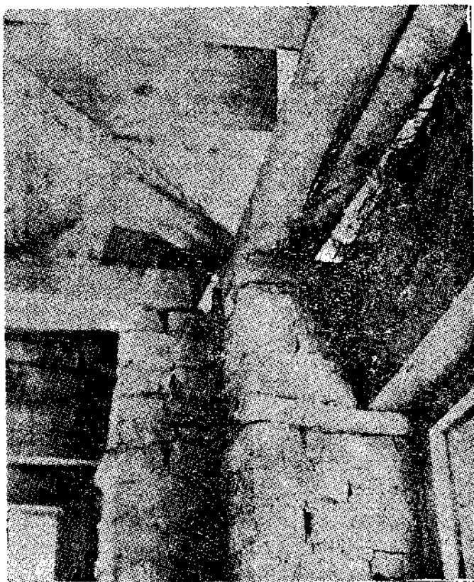
Fig. 21. Wall Plates of Short and Long Walls (Note the absence of connection between the two)
