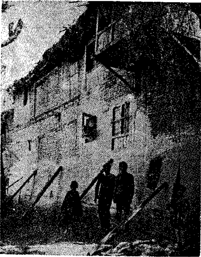
Fig. 7. Timber Rakers supporting out of Plumb Walls
