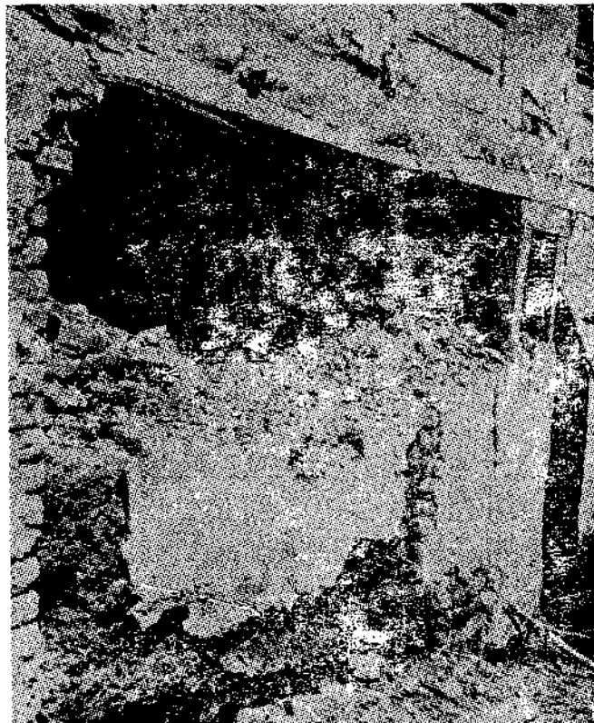
Fig. 11. Damage of Ground Floor Wall made of Adobe, Mud and Muck
