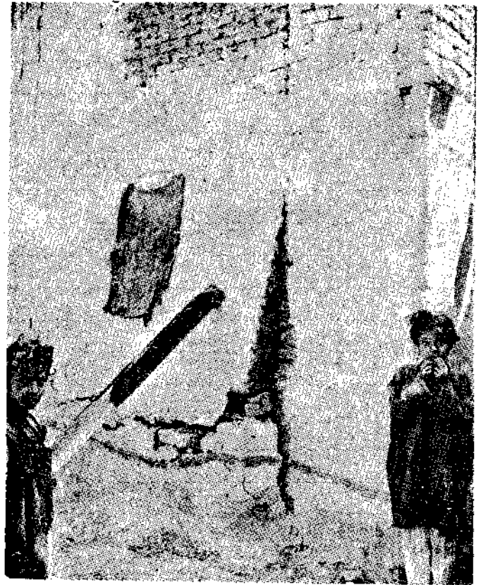
Fig. 8. Close-up of the Damaged Wall shown in Fig. 7
