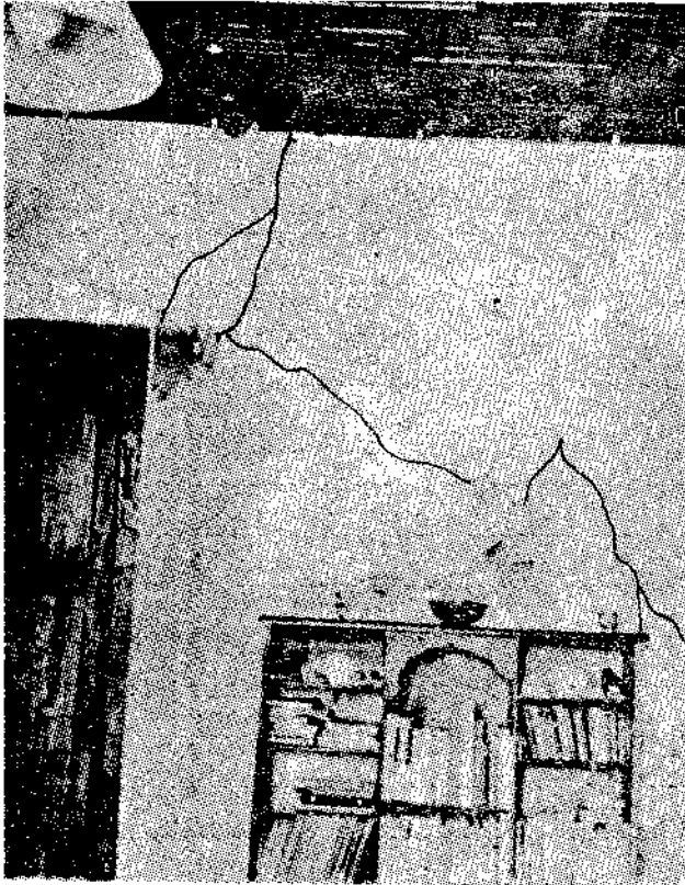
Fig. 27. Diagonal cracking of interior Sun Dried Brick Masonry Wall in Mission Hospital, Anantnag.
