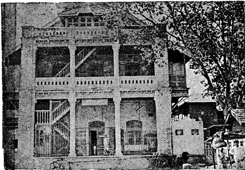
Figure 9. Bharucha Town Hall, Broach, northern view after earthquake.
