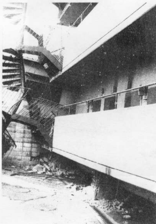
Fig.8 Failure of building due to weak columns (a) super structure (b) failure of columns
