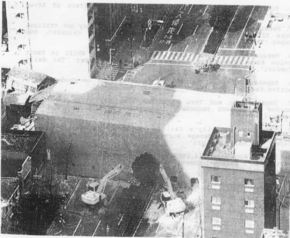
Fig.20 Collapsed building due to aftershocks
