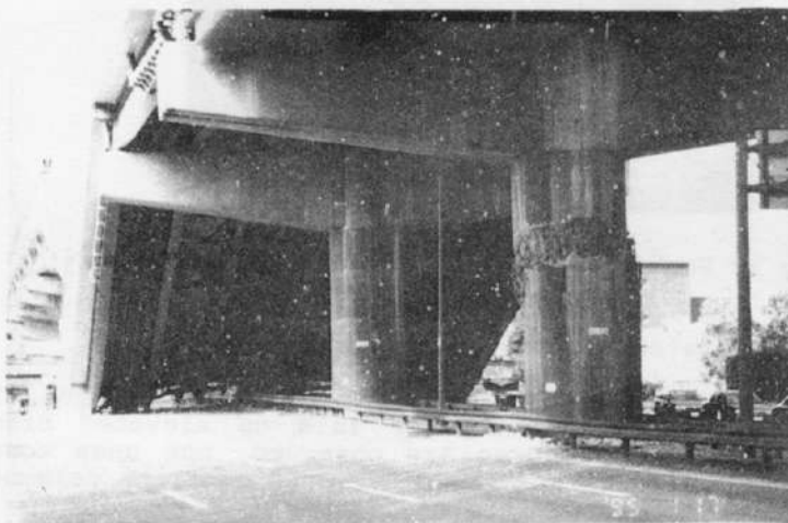
Fig.12 Collapsed bridge girder and typical column failure of Hanshin highway
