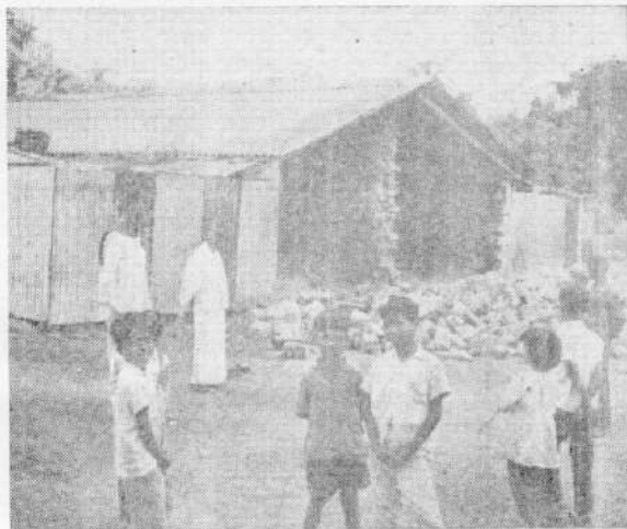
Fig. 11. Stone masonry wall at gable end which suffered extensive damage necessitating its dismantling.
