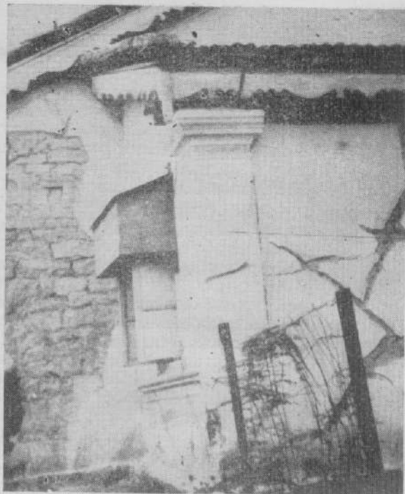
Fig. 5. Development of cross fracture and radial cracks in the wall and rupture of the masonry pillar on the east gable end side of Shri M. C. Ramasamy's residence. Cracks from window sill level extend down towards foundation.
