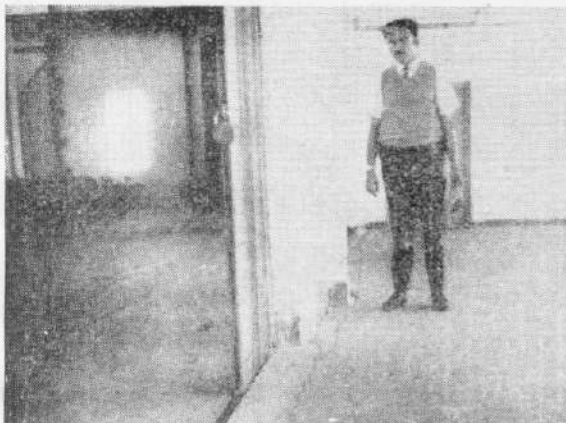
Fig. 23. Development of a crack in the floor near the 10.5 m high southern wall of the Tool Room Shop of Bharat Earth Movers Ltd. which propagated parallel to the length to the wall in all the rooms.
