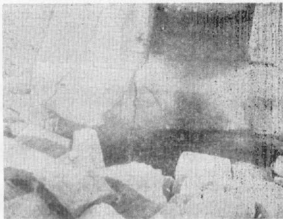
Fig. 19. The concrete foundation of the back brace of the head frame of the Henry's shaft which developed extensive cracks.
