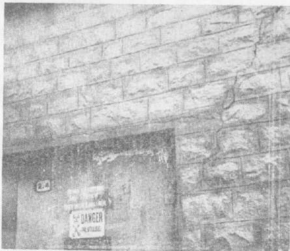
Fig. 16. Development of cracks in stone masonry north wall of the Lighting Sub-Station in Henry shaft area. Similar cracks developed in other walls of the structure.
