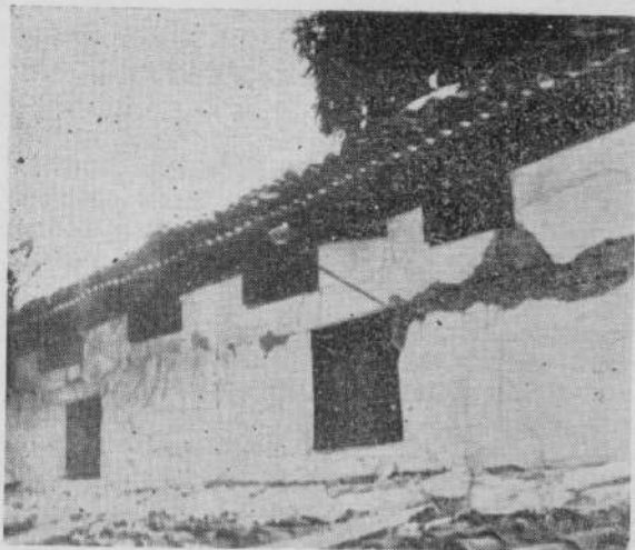
Fig. 3. Cracks in western wall near roof level, extending from window and ventilator openings at Shri A. C. Hiriannah's residence.
