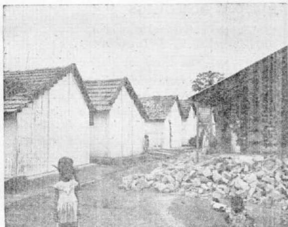
Fig. 12. End wall of stone masonry row house which suffered extensive damage with partial collapse of masonry, necessitating dismantling part of the wall, whereas prefabricated reinforced concrete houses in the left did not suffer any damage.
