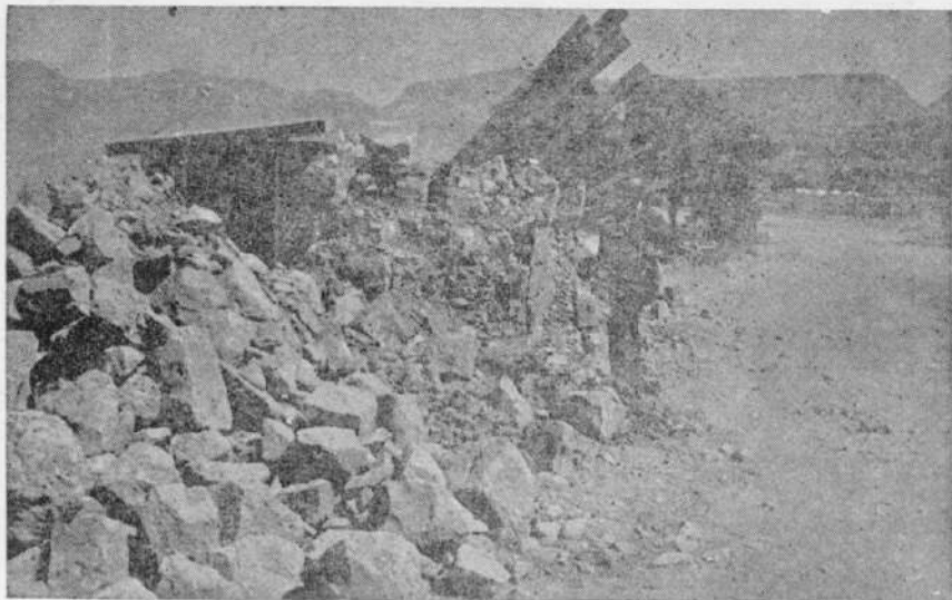
Photo 3. Complete Collapse of a single storied dwelling of random stone construction near Dohran.
