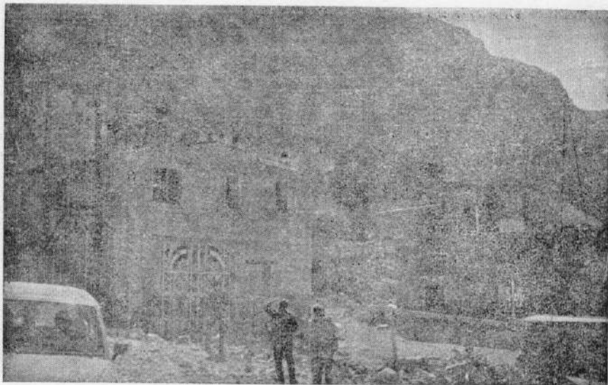
Photo 31. Electrical substation building, minor crack in wall in village Dohran (Dressed stone masonry in cement mortar).
