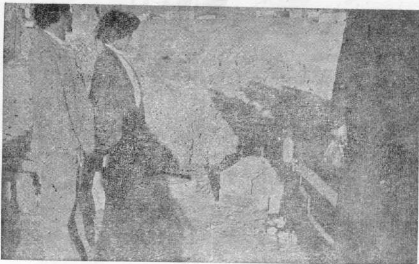
Photo 25. Adobe making in progress in village Al-Olayb. Corner wall construction shown size of adobe is such that breaking of vertical joints in different courses is perfectly arranged.
