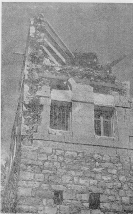
Photo 8. Collapse of third storey and cracks in lower storey walls, very heavy floors in houses seen in village Dohran.
