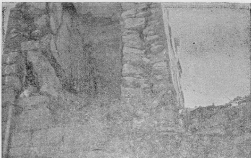
Photo 13. Random rubble stone wall, no interlocking between inner outer faces of stones at Village Hizrat Mangada.
