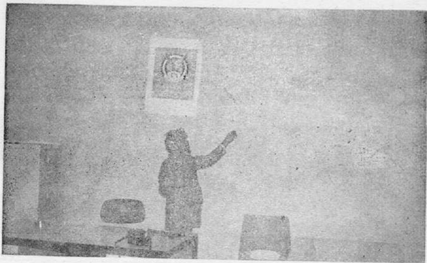
Photo 34. Diagonal cracks in the wall (inside view) in a room of the Dohran Dispensary, stone masonry consisting of half-dressed stones built in gypsum mortar.
