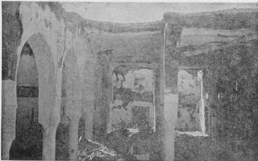
Photo 11. Damages to the Dohran Madarsa-cum-Mosque, fallen wood pieces from roof, cracked and peeled off plaster on walls and pillars.
