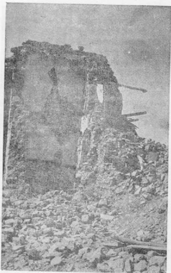
Photo 6. Complete Collapse of a house of random stone construction with muck filling in the hearting of walls at village Dohran.
