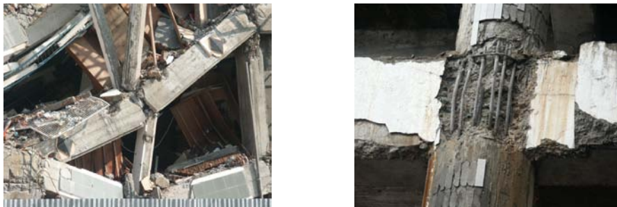
(a) Failure of beam-column connections (b) Lack of joint reinforcement
