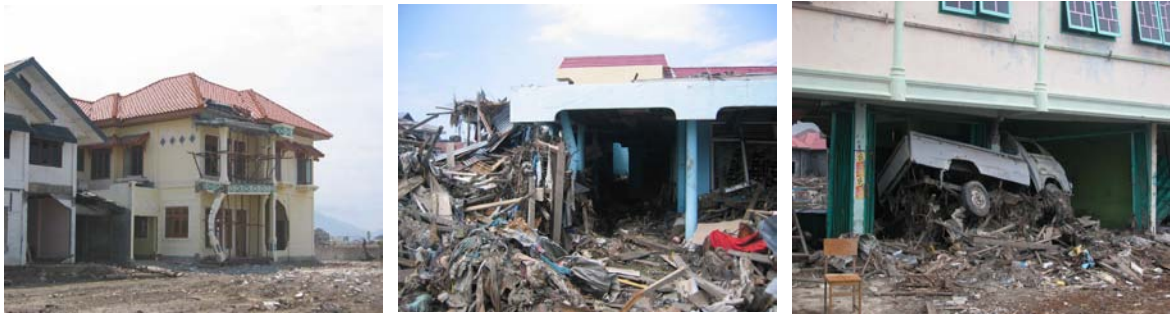
Fig. 18 Column failures due to debris impact in Banda Aceh
