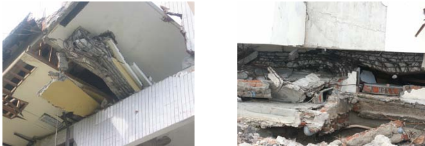
(a) Column failure in Tax Office (b) Column failure in Customs Building
