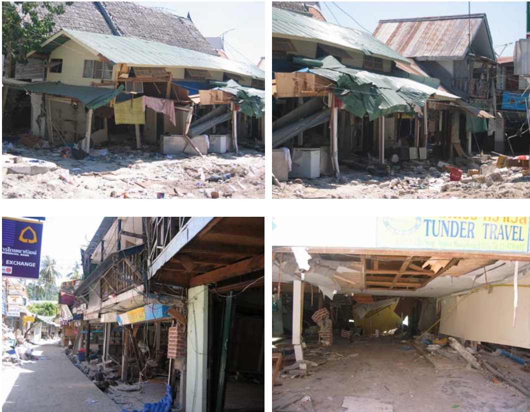
Fig. 14 Damage to timber frame buildings in Phi Phi Island, Thailand
