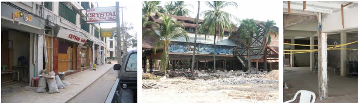
Fig. 5 Damage in Patong Beach
