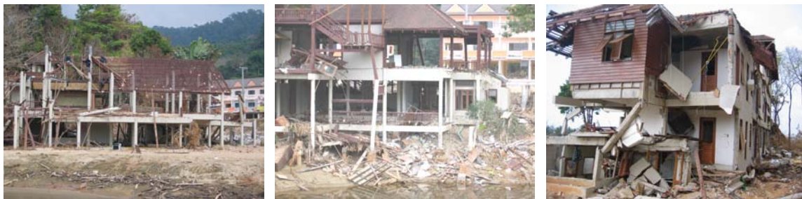
Fig. 6 Structural damage in Nai Thon Beach due to tsunami waves
