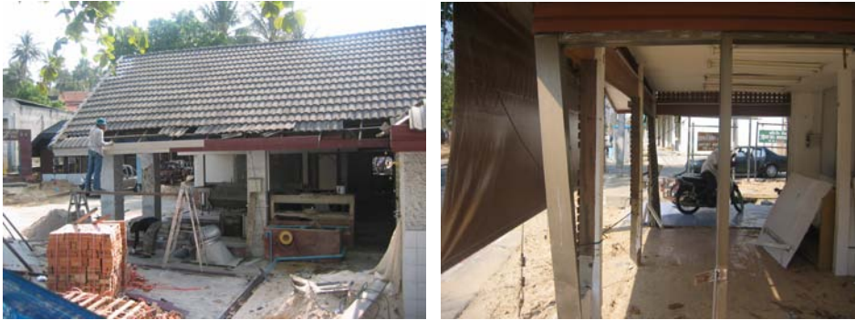
Fig. 4 Damage to single story non-engineered buildings in Kata Beach
