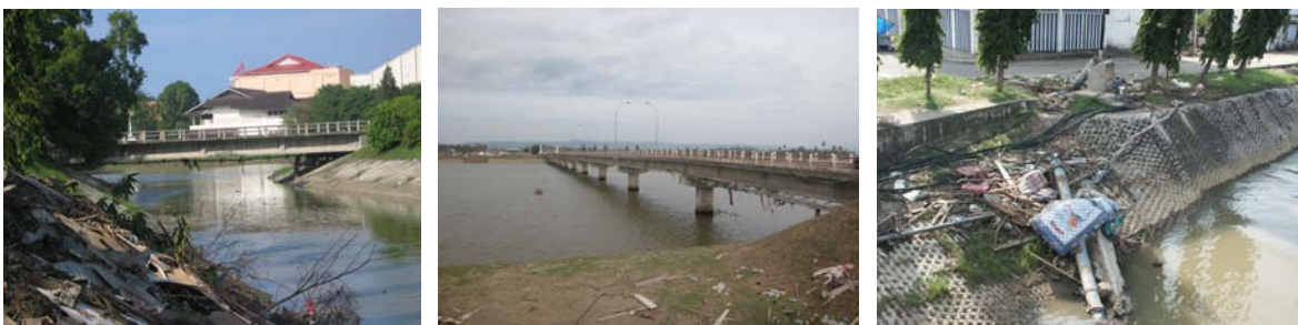
Fig. 26 Damage to pipeline attached to the underside of bridge girders in Banda Aceh
