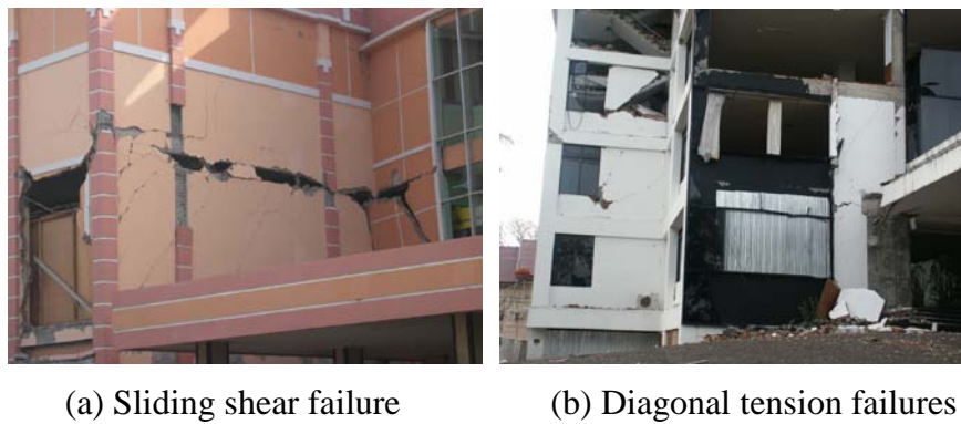
Fig. 32 Masonry damage in Banda Aceh
