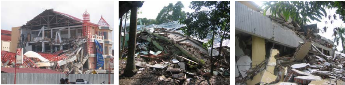
Fig. 11 Earthquake damage in Banda Aceh, Indonesia
