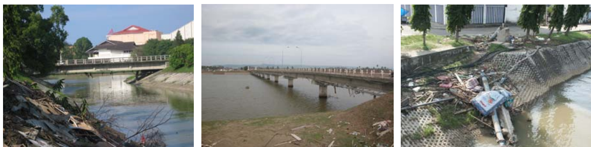
Fig. 26 Damage to pipeline attached to the underside of bridge girders in Banda Aceh
