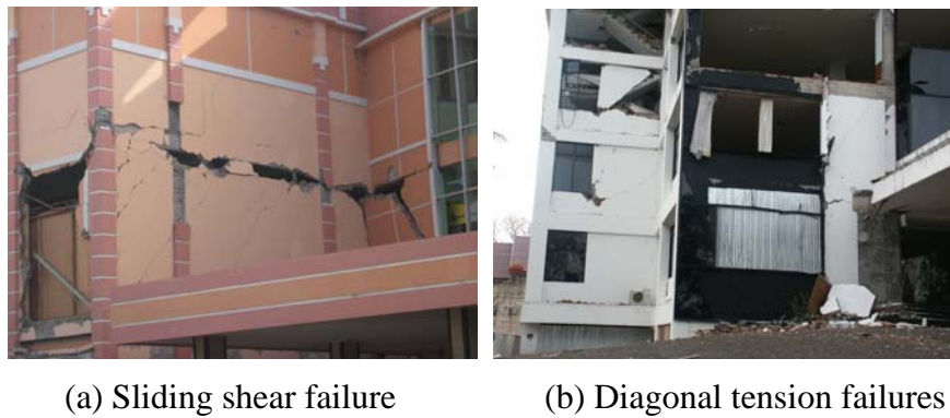
Fig. 32 Masonry damage in Banda Aceh
