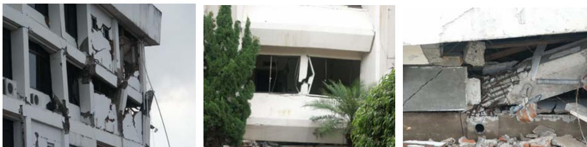
(a) Column shear failure (b) Column shear failure (c) Splice failure
