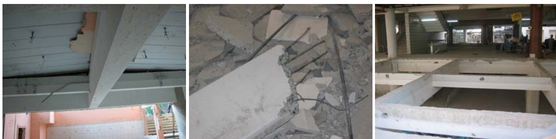
Fig. 20 Failure of precast slab strips in Patong Beach
