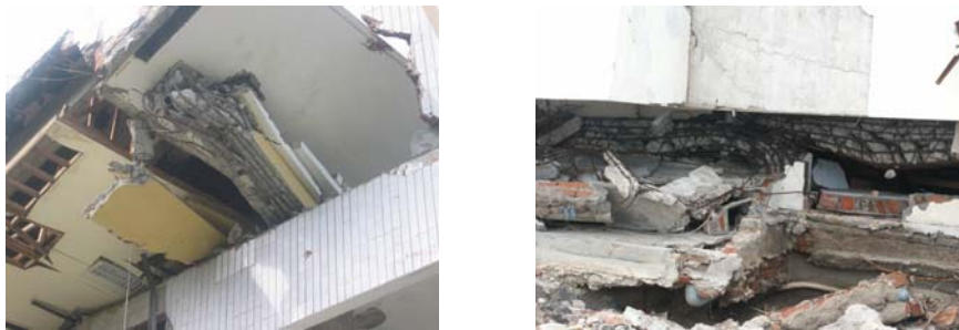
(a) Column failure in Tax Office (b) Column failure in Customs Building
