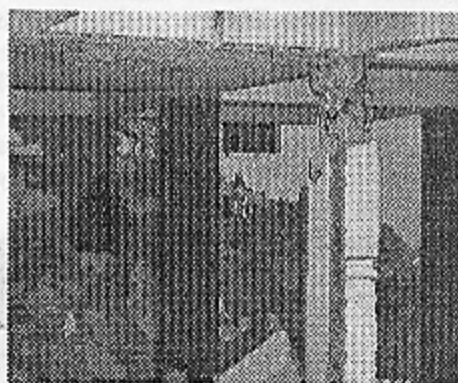
(a) Cracking and spalling of concrete in first storey column
