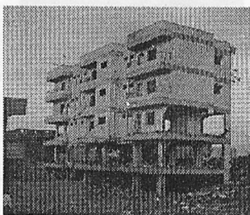
(b) Damage to walls of ground and first floor
