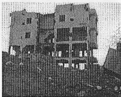
(a) Collapse of exterior wall due to restricted ductility of concrete frame
