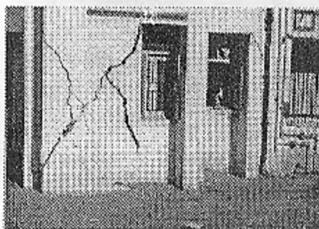
(a) Shear (X) cracking of masonry infill
