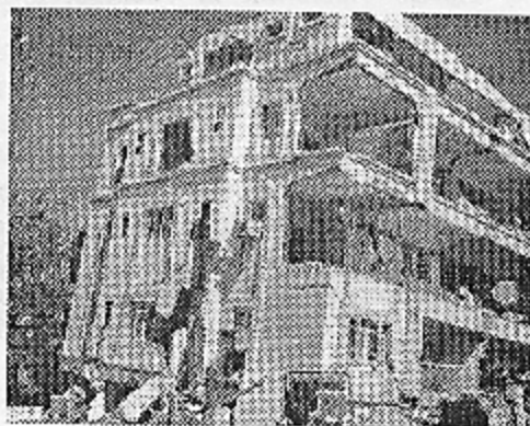
(b) Nilima Park Apartment, Ahmedabad; large scale damage in the upper floors
