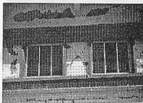
(b) Shear failure in "captive column"
