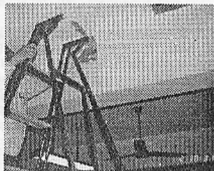
(b) Cracks at slab-beam junction
