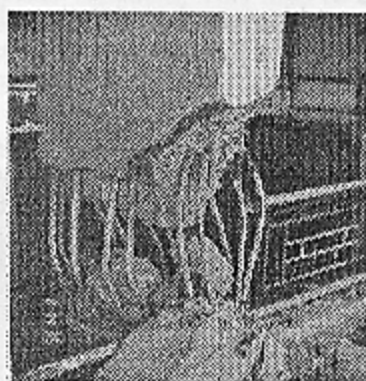
(b) Base of first storey column with widely-spaced ties and spalled concrete
