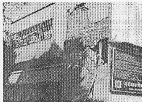
(b) Poor quality of material, corrosion of reinforcement
