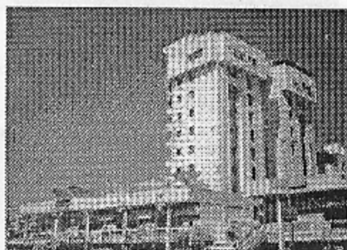
(b) Collapse of A-Block of Mansi Complex while B-block suffered minor damage
