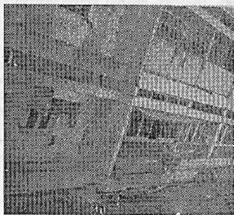
(a) Apollo Apartment at Ahmedabad; ground floor completely collapsed
