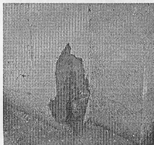
(b) Damage due to corrosion of steel at column face
