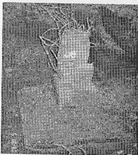
(d) Exposed isolated footing of a column of Shikhar Apartment, Ahmedabad
